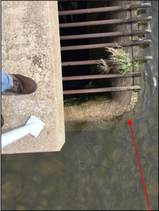
Spalling and Cracked Concrete
